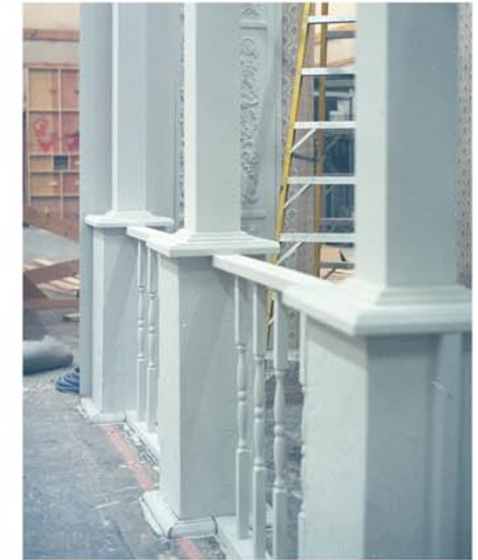
Above: The cabin on stage 6 at various stages of completion Above Right: Ford's Theater Box- mid construction.
